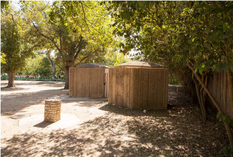
Pecan Grove Picnic Area: The existing restrooms at the Pecan Grove Picnic Area are in poor physical condition.
