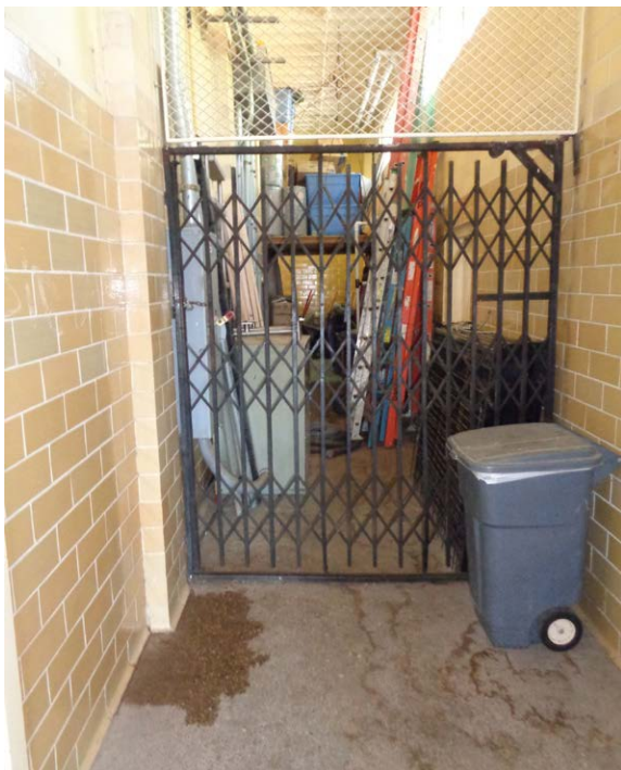
Bathhouse Men's Changing Area – Entry Corridor: This corridor is used both for storage (including the incorporation of an improvised mezzanine) and for the location of portions of the electrical service for the Bathhouse.
