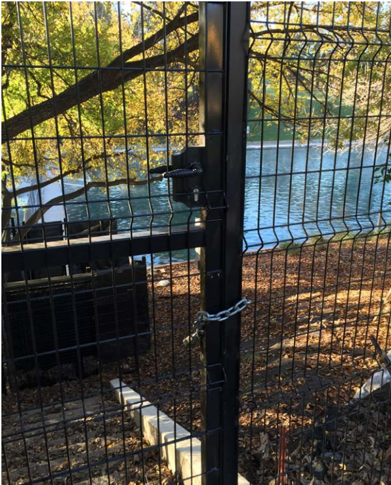
Pool Enclosure: Emergency egress from the pool enclosure is a matter of significant concern. Exits from the enclosure do not comply with current code requirements, a deficiency compounded by features such as locked gates.
