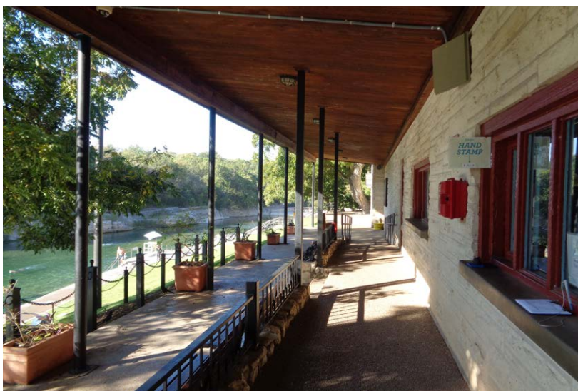
Bathhouse Spectators' Gallery: The Spectators' Gallery serves as the principal means of access to and from the north side of the pool. The Gallery was not intended for this purpose.
