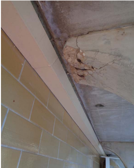
Bathhouse Men's Changing Area: The concrete canopy structures in the mens' and womens' changing areas are in poor condition, with a significant percentage exhibiting spalling concrete and exposed reinforcing.
