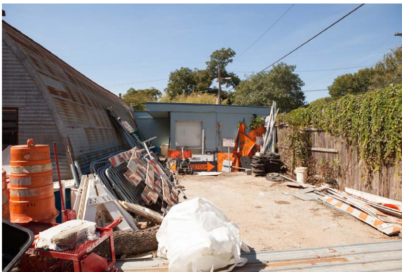
Maintenance Yard: The Quonset storage building, although an interesting structure, has reached a serviceability limit state. The extent of rust visible on the exterior of the building, and the number of open holes visible from the interior, indicate a building past economic rehabilitation. It would be less expensive to replace this building than it would to repair it for a different use.
