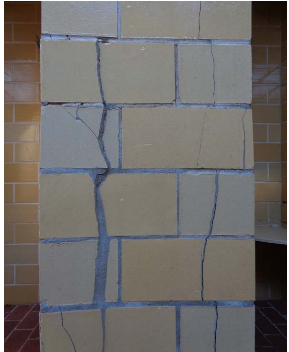
Bathhouse Men's Changing Area: A typical example of structural deterioration of the glazed structural tile partitions in the mens' and womens' changing areas. This appears to be the consequence of a flaw in the original building design, which did not include dedicated foundations for these partitions.
