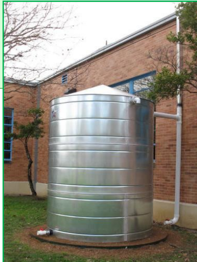
Rainwater tank at Zilker school
