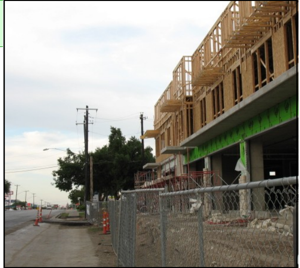
Construction near the Broken Spoke and a future traffic light on South Lamar. The gray point at the end of the sidewalk is the Capitol dome. Changes to Austin's roadway design criteria and their effect on South Lamar will be presented at the ZNA Quarterly Meeting on May 20.
