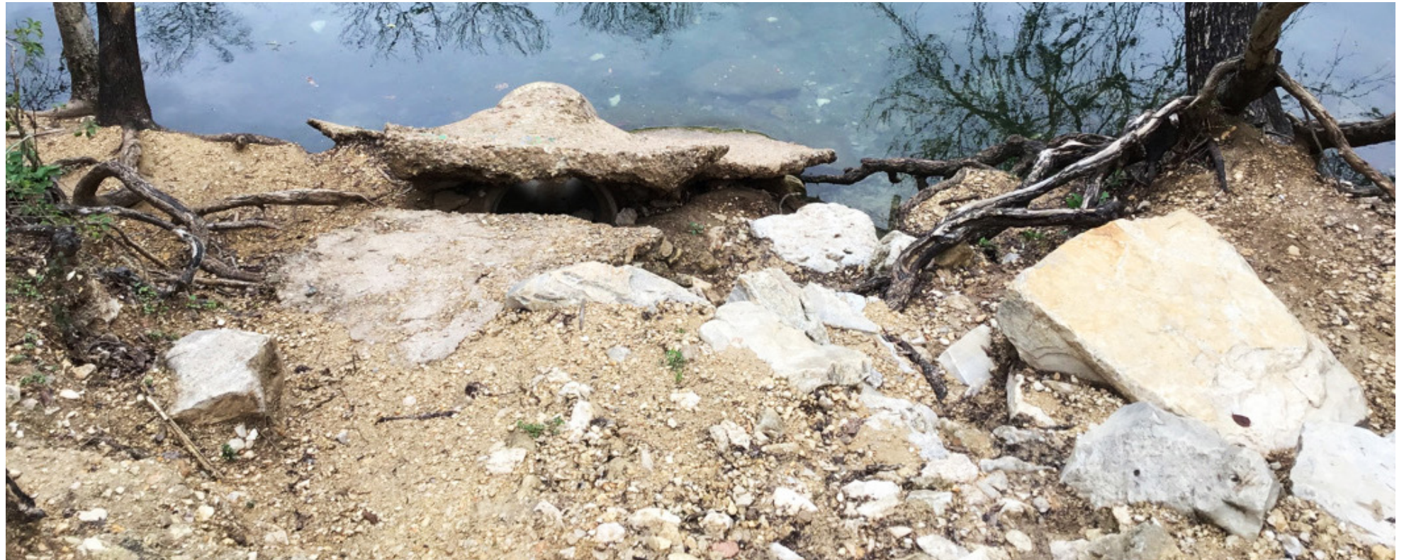
Decomposed granite decomposition near water edge
